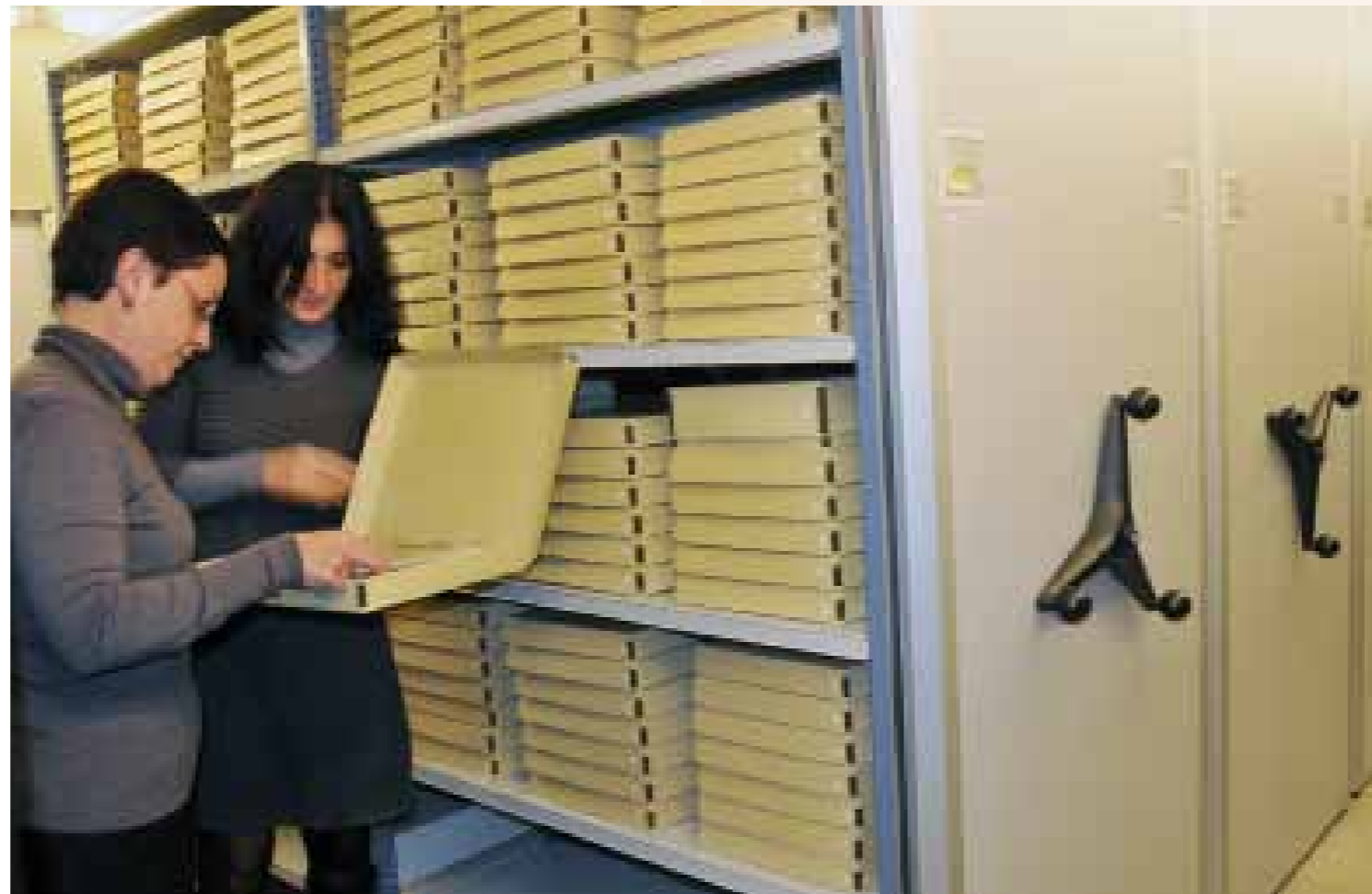
The CED has installed mobile shelves in the new office building Le CED dispose de rayonnages mobiles dans le nouvel édifice de bureaux
